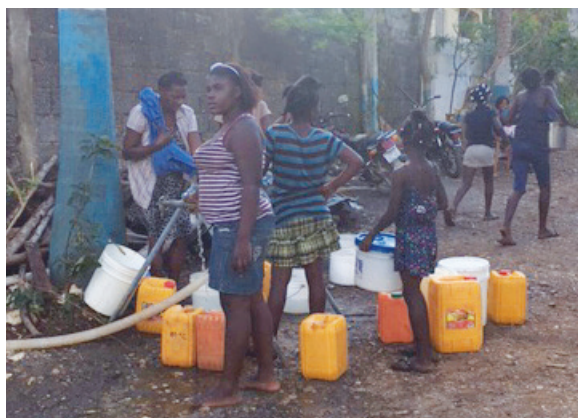
Villagers getting water from newly installed / repaired central water system. Sea water breached the sea wall and came in so far during Hurricane Matthew that fresh water supplies were contaminated.
